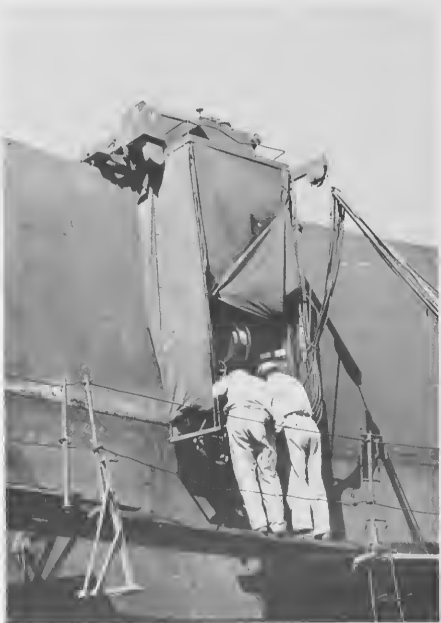
ONE OF the fascinating devices used in building the tanks is the auto- matic welding machine that looks like a voting booth, runs like a trolley and welds horizontal seams faster and straighter than a crew of men. UN DI e aparatonan fascinante usá den construccion di tankinan ta e mashien automatico di welding, cu ta parece manera un urna electoral, ta corre manera un trolley y ta weldo seams horizontal.
